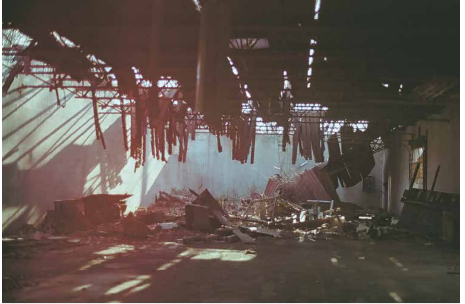
Abandoned An abandoned brass mill in my town makes for some nice walks through now and then. This building caught fire at some point. The film gave a nice array of colors with the exposure.
