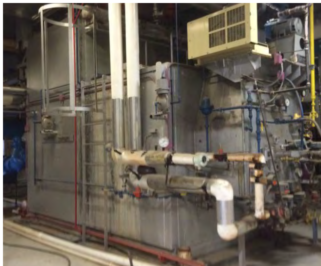
Boiler in Central Plant
